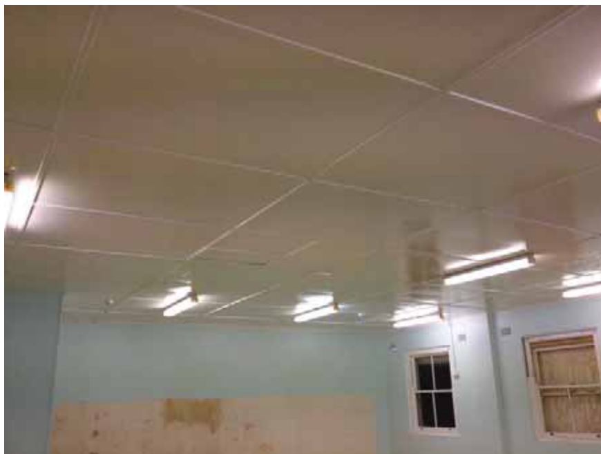
Photograph 16 – Building 10, Presumed asbestos containing flat sheet interior ceiling lining
