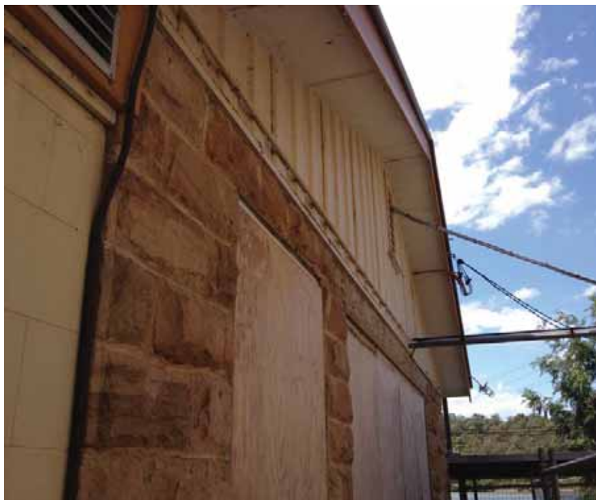
Photograph 02 – Building 2, Asbestos containing flat sheet eaves and fascia cladding
