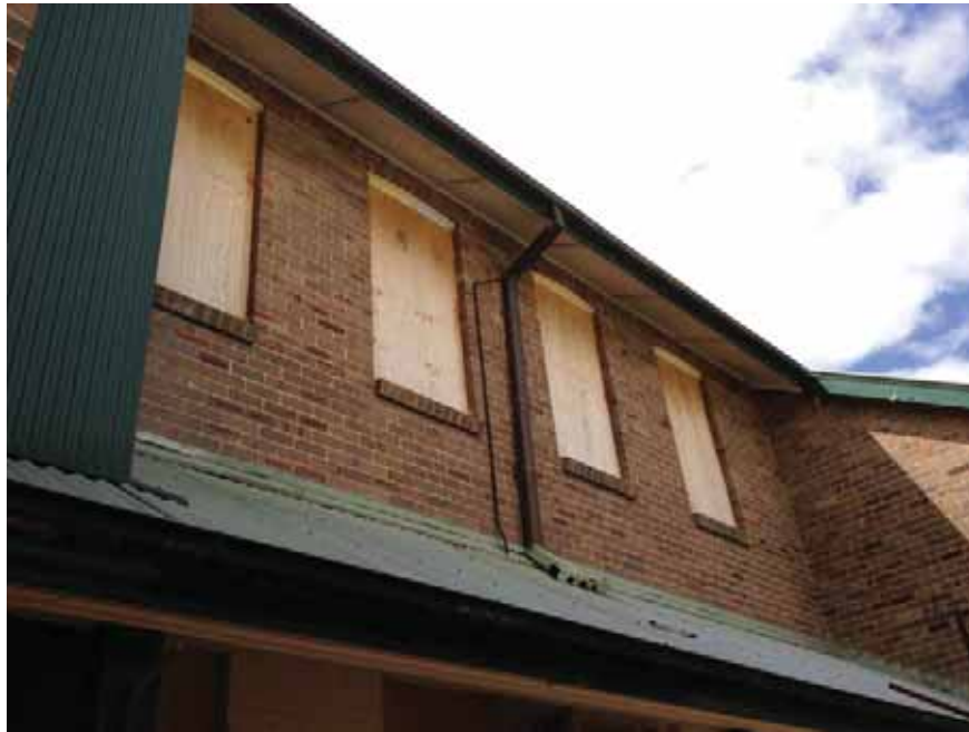
Photograph 19 – Building 11, Presumed asbestos containing flat sheet eaves
