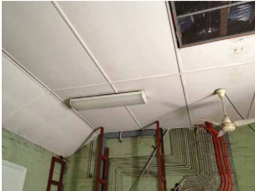
Photograph 13 – Building 9, Asbestos containing flat sheet ceiling lining in utility room.
