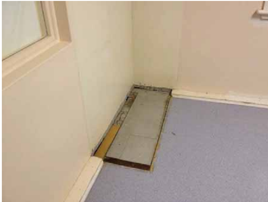
Photograph 21 – Building 11, Asbestos containing vinyl floor tiles beneath office area cupboards on first floor
