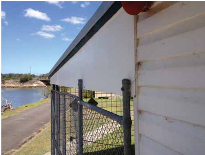
Photograph 03 – Building 3, Asbestos containing flat sheet garage fascia board
