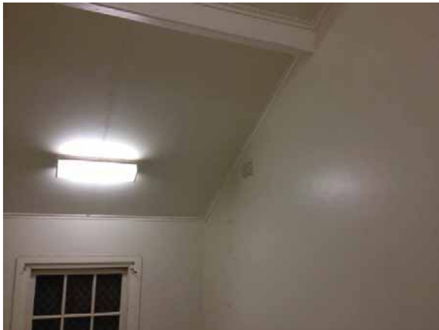
Photograph 22 – Building 11, Presumed asbestos containing flat sheet stairwell ceiling lining
