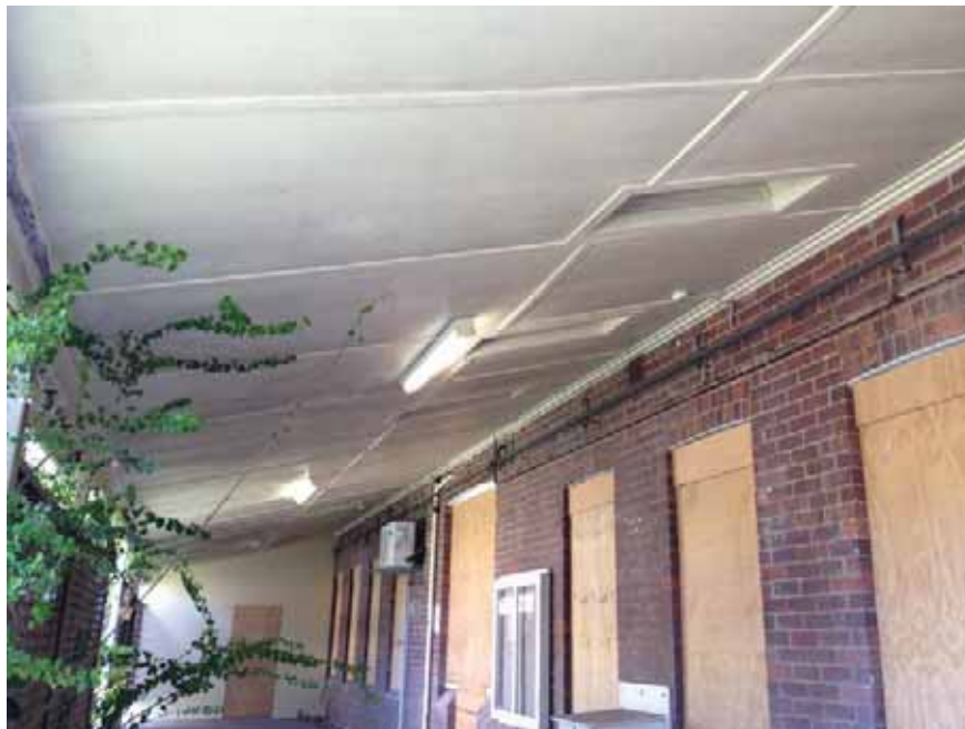
Photograph 04 – Building 4, Asbestos containing flat sheet porch ceiling lining
