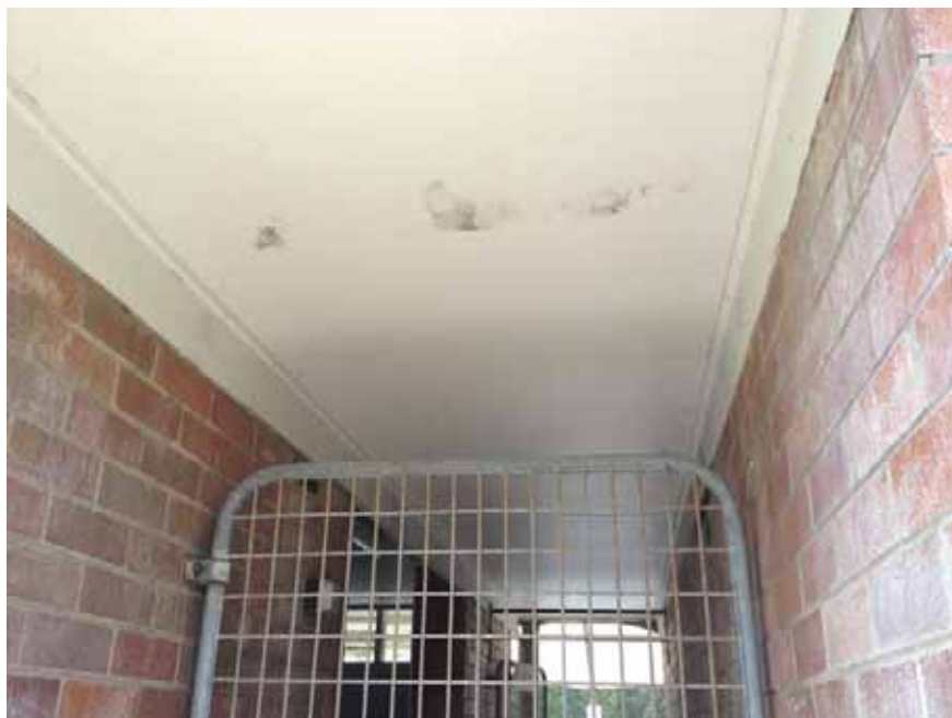
Photograph 28 – Building 18, Asbestos containing flat sheet ceiling lining
