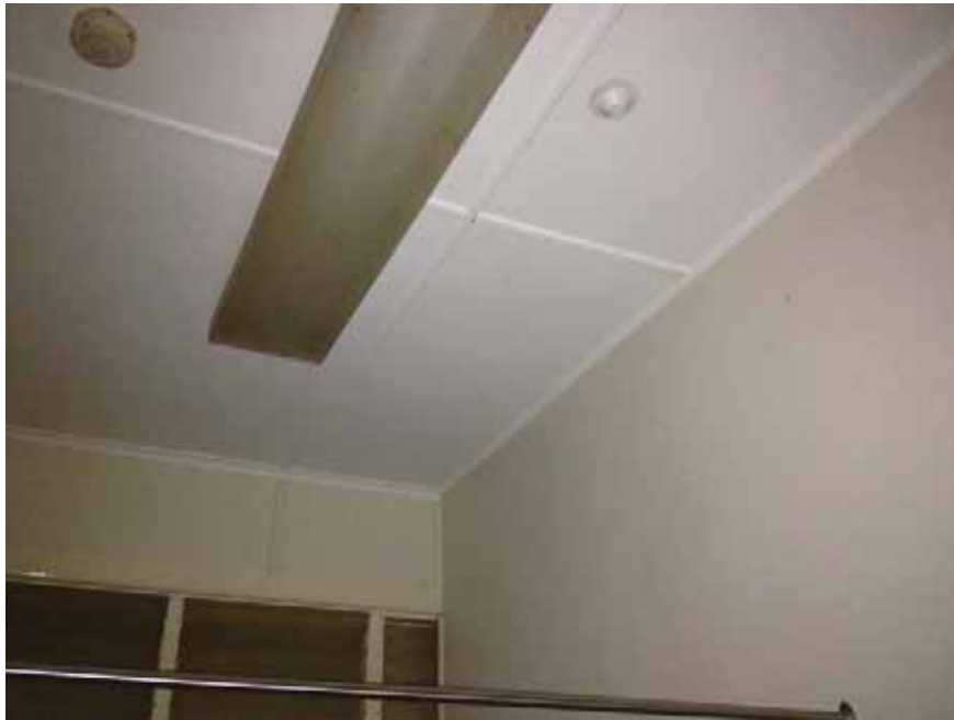
Photograph 01 – Building 1, Asbestos containing flat sheet ceiling lining within interior shower rooms
