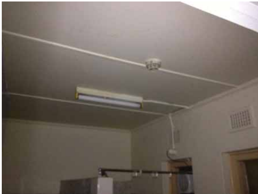
Photograph 08 – Building 5, Presumed asbestos containing flat sheet ceiling lining in ground floor (southern) bathroom
