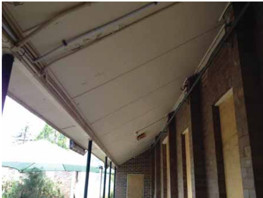
Photograph 06 – Building 5, Presumed asbestos containing flat sheet porch ceiling lining
