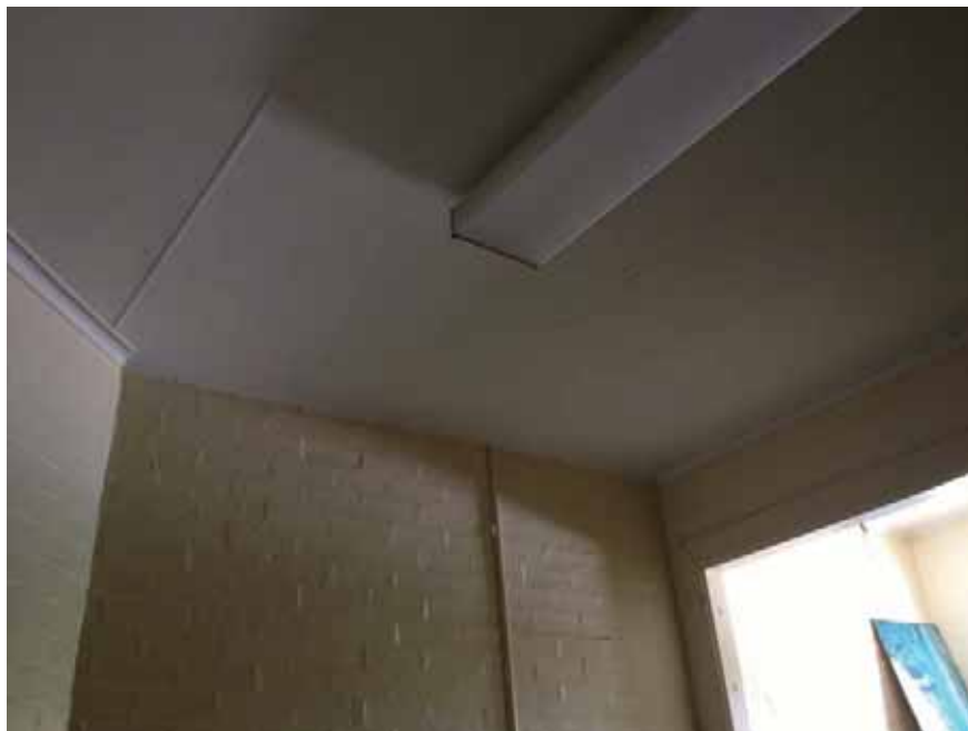
Photograph 26 – Building 14, Asbestos containing flat sheet ceiling lining
