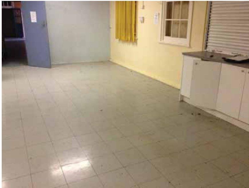
Photograph 9 – Building 5, Asbestos containing vinyl floor tiles in kitchen
