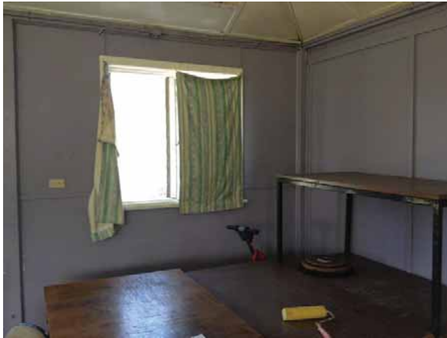
Photograph 29 – Building 20, Presumed asbestos containing flat sheet wall lining
