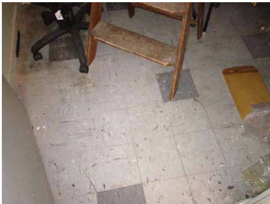
Photograph 14 – Building 9, Asbestos containing vinyl floor tiles in utility room
