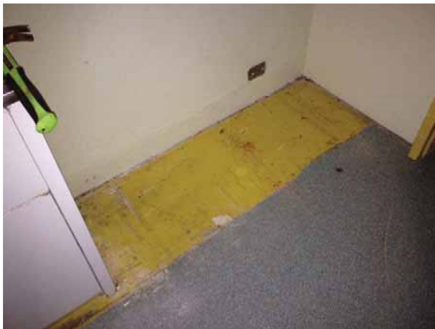
Photograph 12 – Building 6, Asbestos containing vinyl floor tiles in laundry
