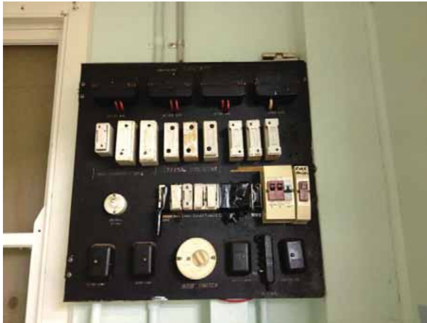
Photograph 17 – Building 10, Presumed asbestos containing 'zelemite' backing board
