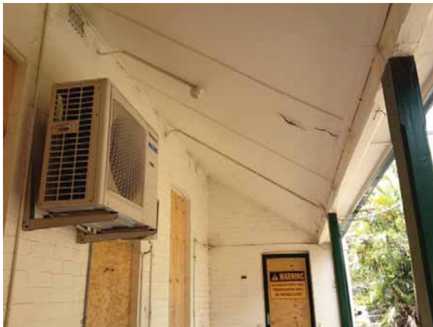
Photograph 20 – Building 11, Asbestos containing flat sheet porch ceiling lining
