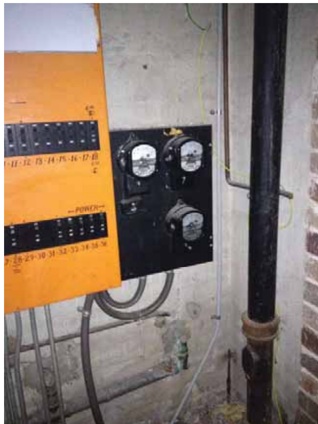
Photograph 34 – Nurses Dormitory, Asbestos containing 'zelemite' backing board (ground floor)
