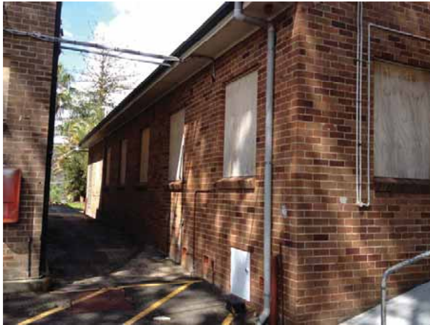
Photograph 15 – Building 10, Presumed asbestos containing flat sheet eaves
