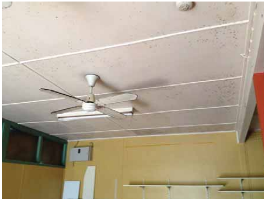
Photograph 32 – Service station, Asbestos containing flat sheet ceiling lining
