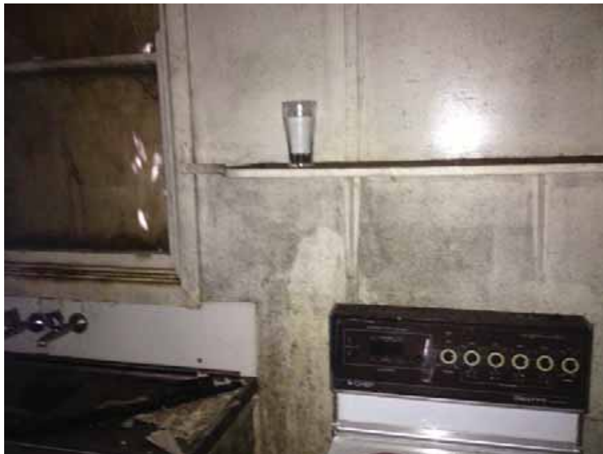
Photograph 30 – 65 Kowan Rd, Asbestos containing wall lining in kitchen
