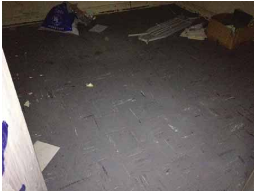
Photograph 25 – Building 13, Asbestos containing blur vinyl floor tiles
