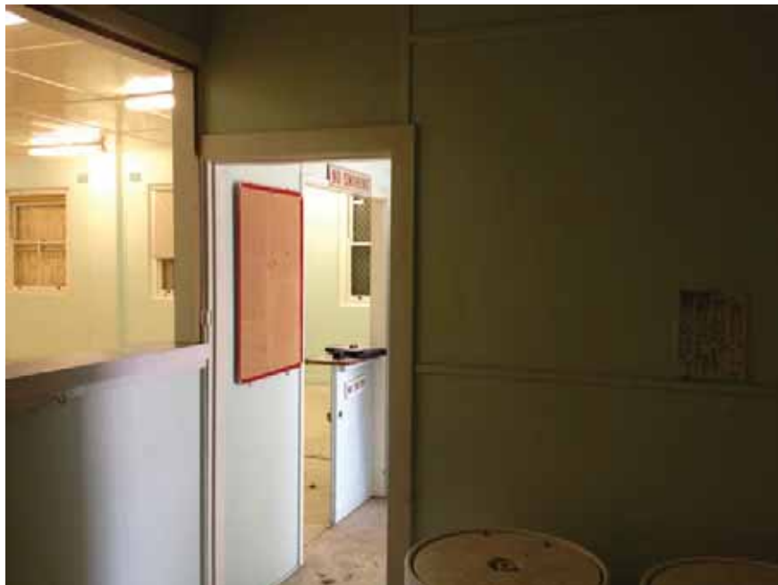
Photograph 18 – Building 10, Asbestos containing flat sheet wall linings
