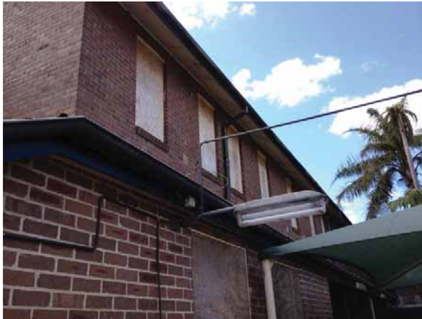
Photograph 07 – Building 5, Presumed asbestos containing flat sheet eaves
