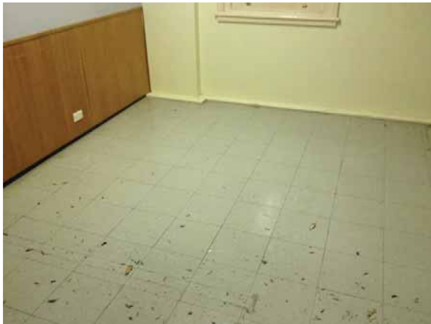
Photograph 24 – Building 12, Asbestos containing first floor vinyl floor tiles
