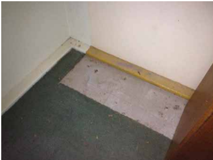
Photograph 10 – Building 5, Presumed asbestos containing vinyl floor tiles beneath carpet in first floor office areas
