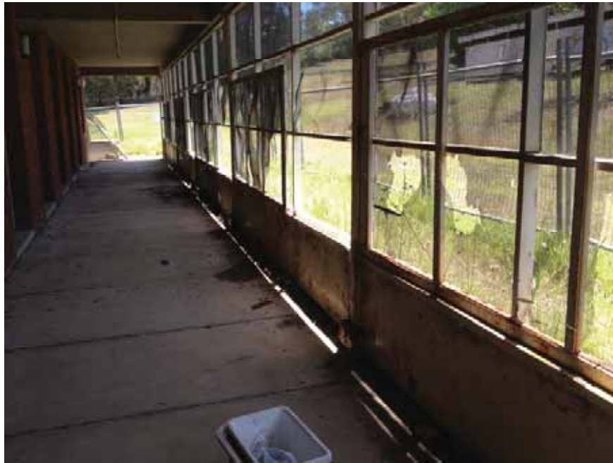
Photograph 33 – Nurses Dormitory, Asbestos containing flat sheet in fill panels beneath porch windows
