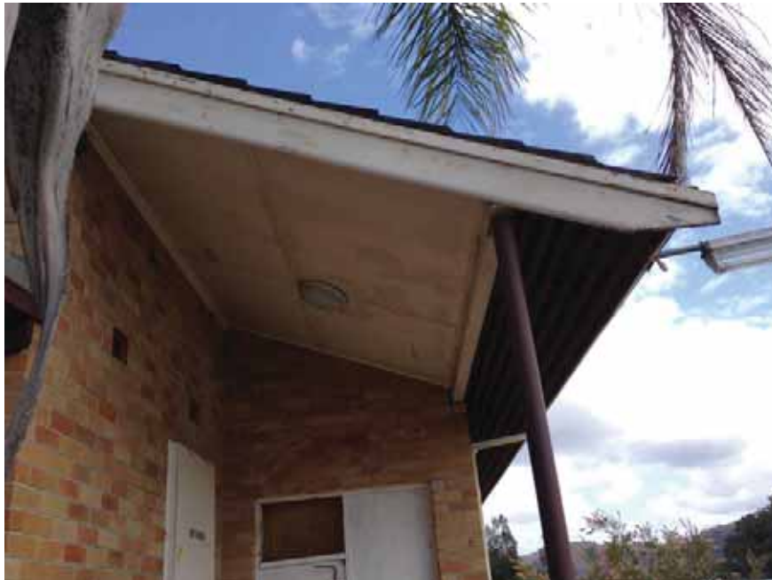
Photograph 11 – Building 6, Presumed asbestos containing flat sheet porch ceiling lining (NE corner)
