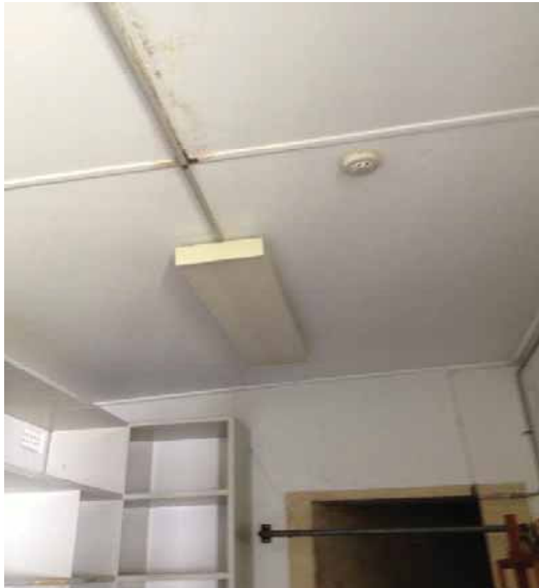
Photograph 05 – Shed adjacent to Building 4, Presumed asbestos containing ceiling lining
